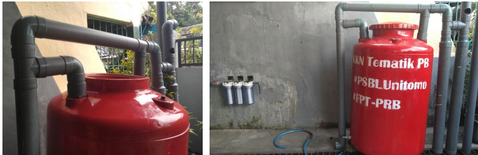
Figure 4. A Series of RHT (Rainwater Harvesting) Installations Complete with Electrolysis
